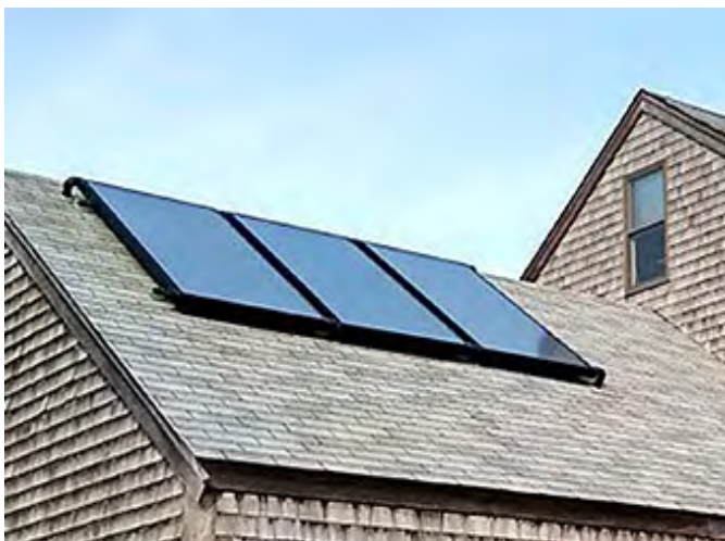
Flat Plate Collector System
