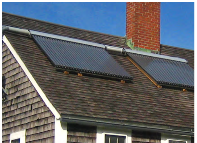
Evacuated Tube Collector System
