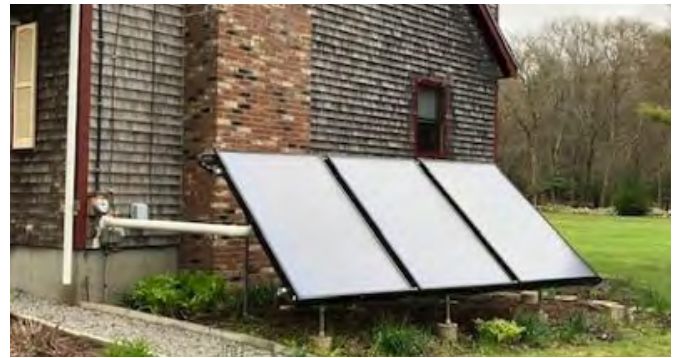
Solar hot water collectors installed on the ground.
