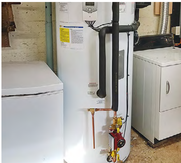
Hot Water Tank
