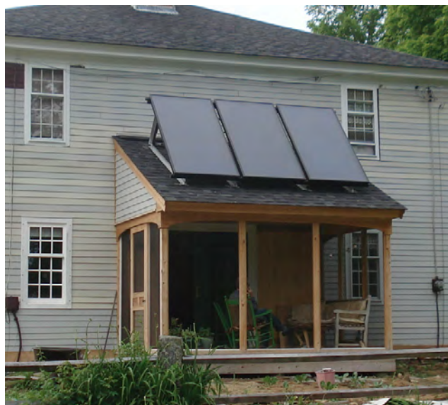
Solar Hot Water Collectors
